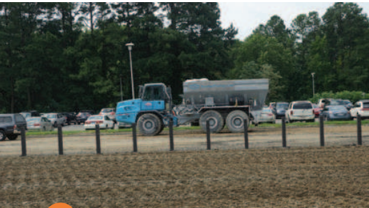
5 The area has been rolled with a padfoot roller to achieve deep compaction. Ruston's precision cement spreader is visible in the background.
