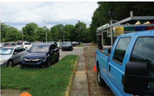
3 Ruston Paving's thoughtful staging and careful construction allowed them to work in close proximity to parked vehicles with minimal disruption.
