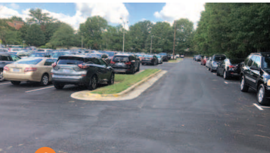
6 Facing the same direction as photo 3, the completed pavement is flush with the preexisting curb-and-gutter and should be trouble-free for years to come.
