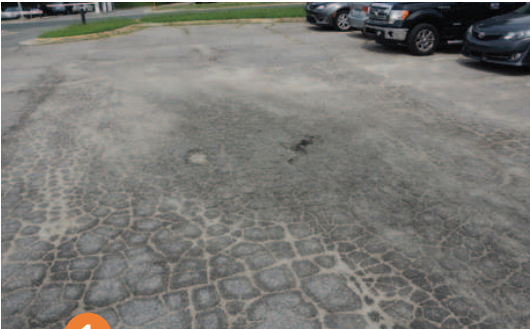
1 Prior to reconstruction with FDR, the parking lot's pavement was in an advanced state of decay.
