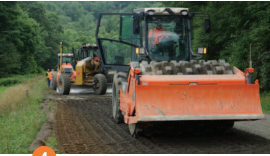
4 Modern reclaiming equipment is highly maneuverable, so working around existing curb and gutter, as well as obstructions such as drop inlets, manholes, and bollards is not a problem. Here, the existing pavement has been pulverized and the reclaimer is mixing a carefully controlled, predetermined amount of cement with the pulverized material.
