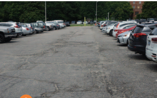
2 Deterioration was widespread, making this site a perfect candidate for FDR. When the need for patching exceeds 15% - 20% of the total area, FDR is often cheaper in initial cost as well as long-term cost.
