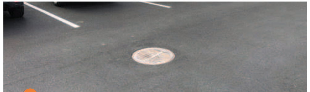
8 Drainage structures in the pavement, such as shown here, and other obstructions can be handled in the FDR process.
