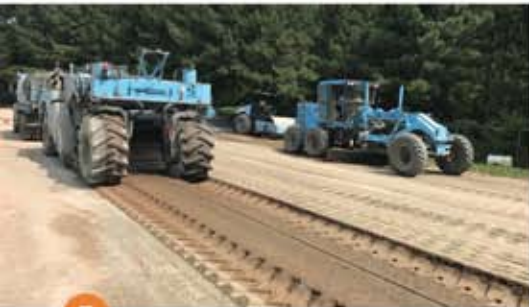
5 As mixing operations continue in the foreground, a motor grader performs fine grading on areas that have been compacted with padfoot roller.
