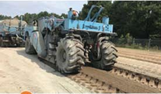
4 Ruston's mixer-reclaimer pushes a water tanker that feeds a precision water injection system to obtain optimum moisture content as the cement is mixed with the pulverized pavement and base.
